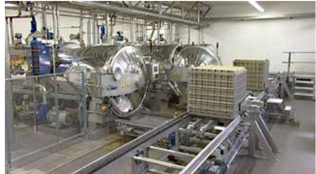
Transport system using fixed conveyors
